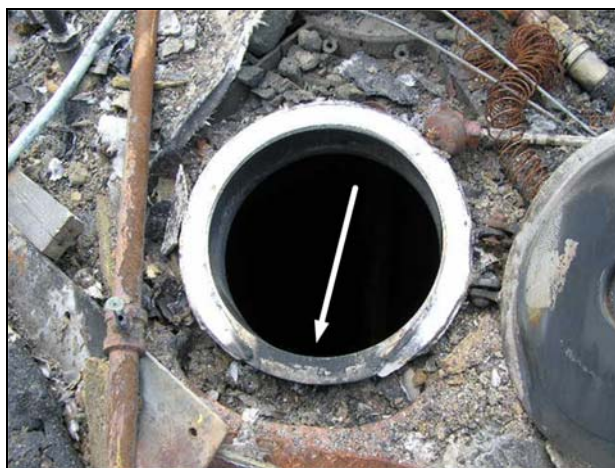
Figure 6. Damaged manway gasket, showing vapor release path
